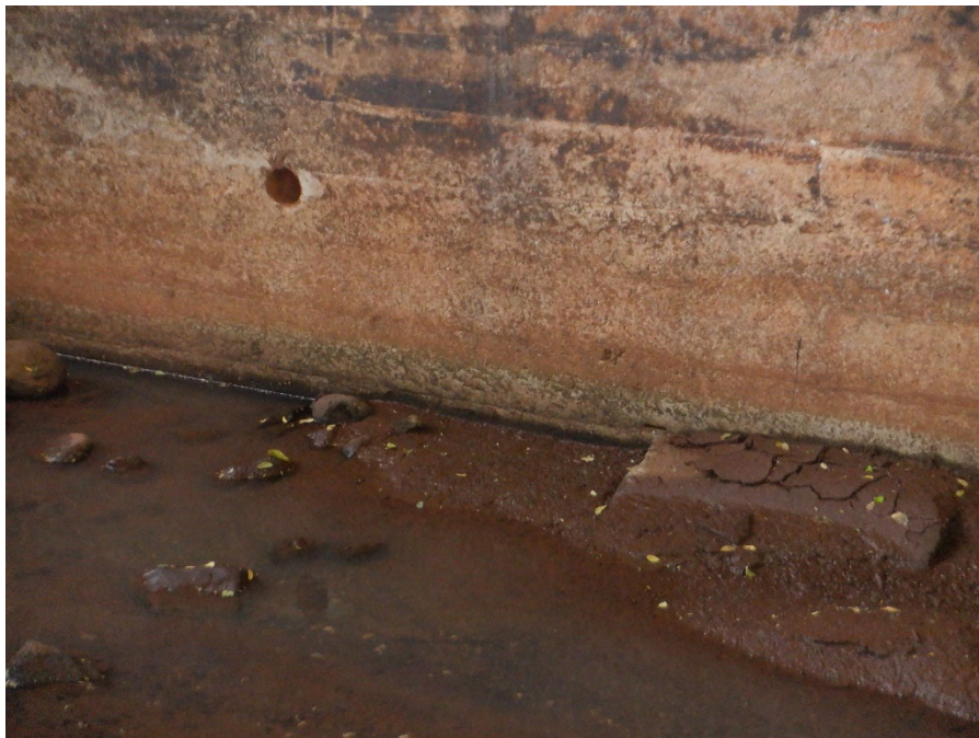
PHOTO 30 PARTIAL ABRASION (1190 CS2) ALONG ENTIRE LENGTH OF ABUTMENT 1 AND WINGWALLS
