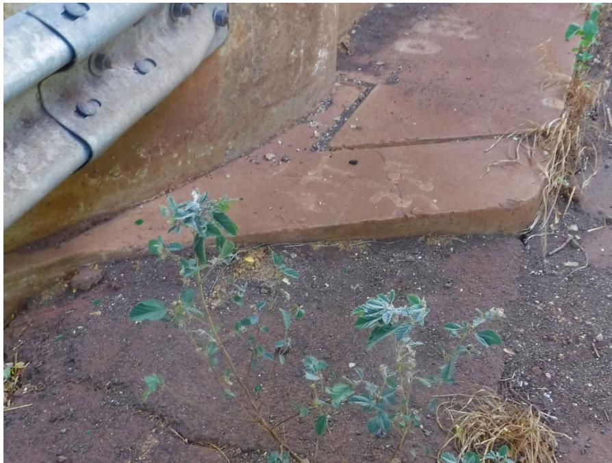
PHOTO 8 3-1/2" VERTICAL DIFFERENTIAL AT WEST APPROACH TO UPSTREAM SIDEWALK
