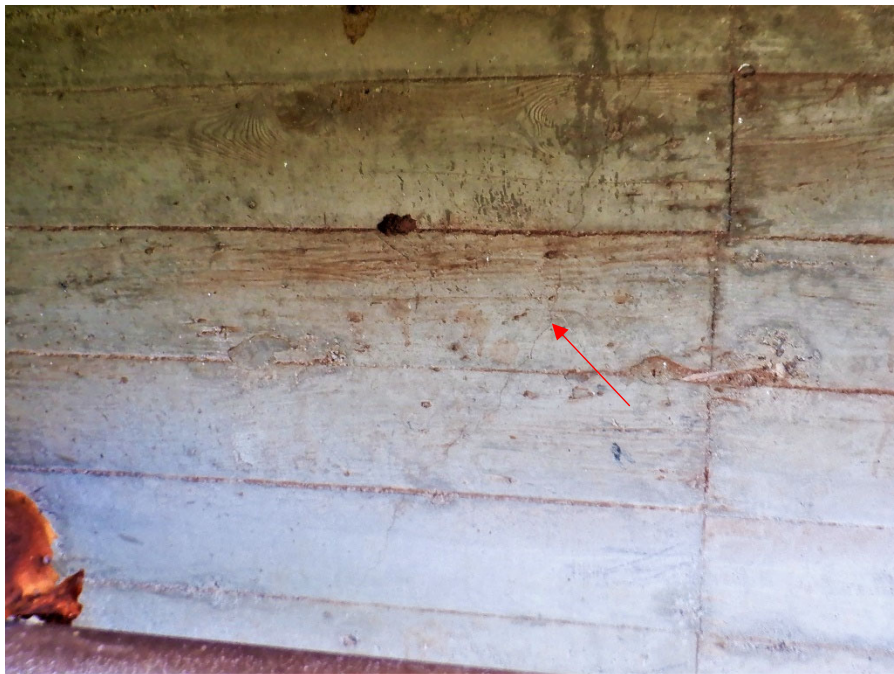
PHOTO 24 TYPICAL MODERATE WIDTH DIAGONAL CRACK (1130 CS2) ON ALL GIRDERS
