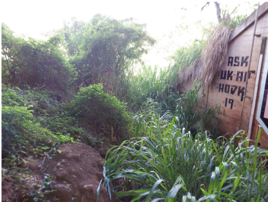
PHOTO 32 UPSTREAM CHANNEL WITH HEAVY VEGETATION GROWTH
