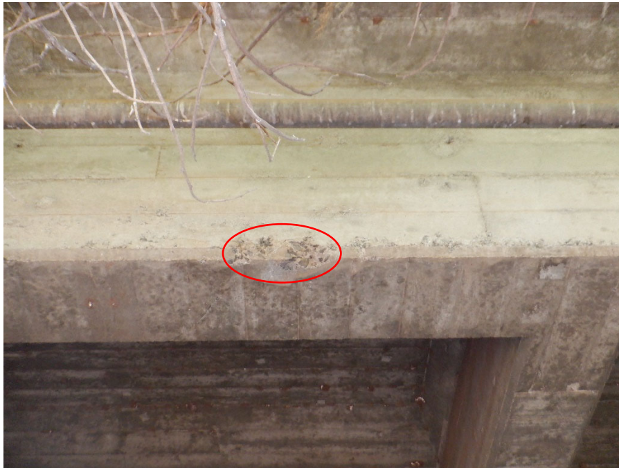
PHOTO 22 6"X2"X2" EDGE SPALL (1FT 1080 CS2) ON GIRDER G4
