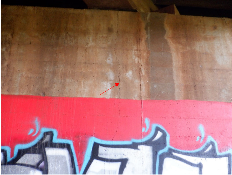
PHOTO 27 WIDE VERTICAL CRACK (1FT 1130 CS3) ON ABUTMENT 2 BELOW GIRDER G2
