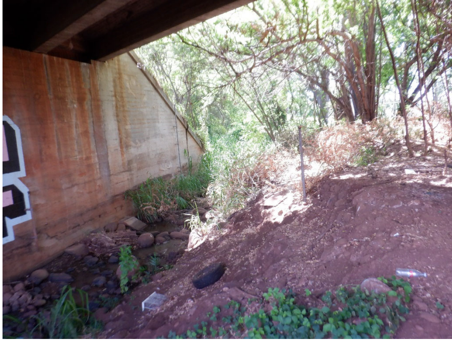
PHOTO 33 DOWNSTREAM CHANNEL WITH VEGETATION GROWTH
