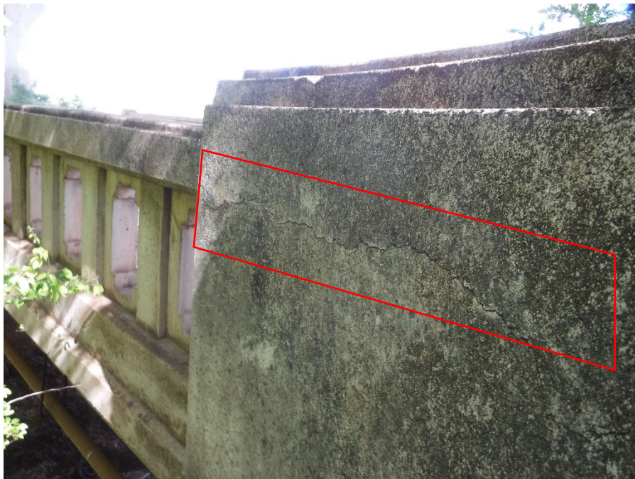
PHOTO 14 4FT LONG HORIZONTAL CRACK AND DELAMINATION (4FT 1080 CS2) ON EXTERIOR FACE OF DOWNSTREAM EAST END POST
