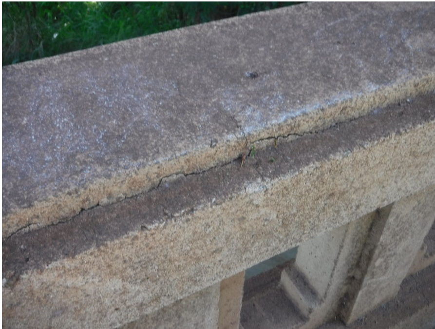
PHOTO 12 TYPICAL DELAMINATION (1080 CS2) ON UPSTREAM TOP RAIL
