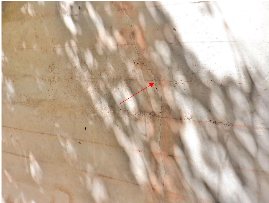
PHOTO 28 WIDE VERTICAL CRACK (1FT 1130 CS3) ON DOWNSTREAM WEST WINGWALL
