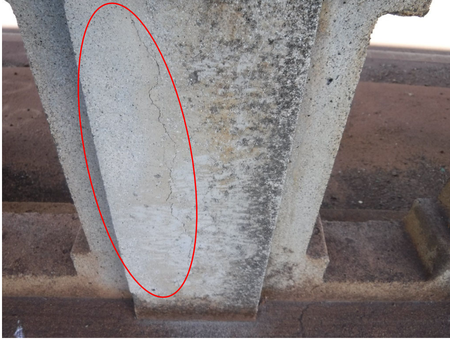
PHOTO 11 TYPICAL DELAMINATION (1080 CS2) ON EXTERIOR FACE OF UPSTREAM RAILING PICKET
