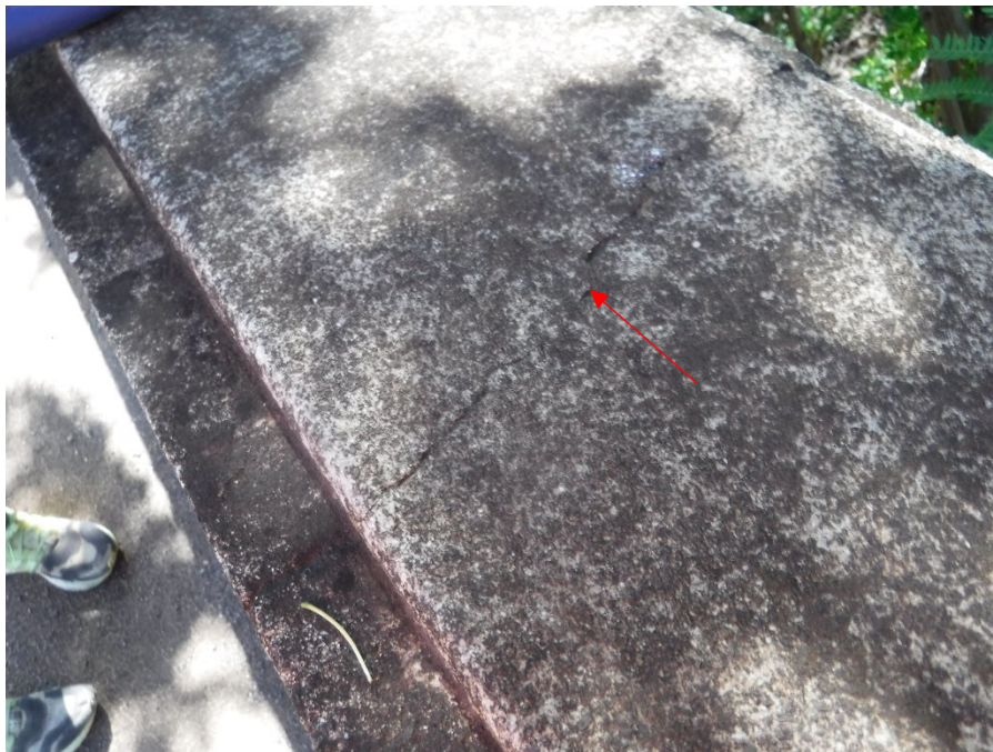
PHOTO 16 TYPICAL MODERATE WIDTH CRACK (1130 CS2) ON BOTH BRIDGE RAILINGS
