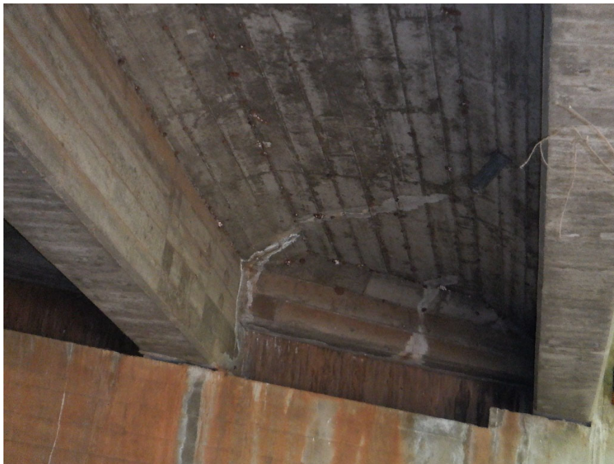
PHOTO 20 MODERATE WIDTH DIAGONAL CRACK WITH EFFLORESCENCE (8SF 1120 CS2) ON TOP FLANGE SOFFIT BETWEEN GIRDERS G3 AND G4 NEAR ABUTMENT 1
