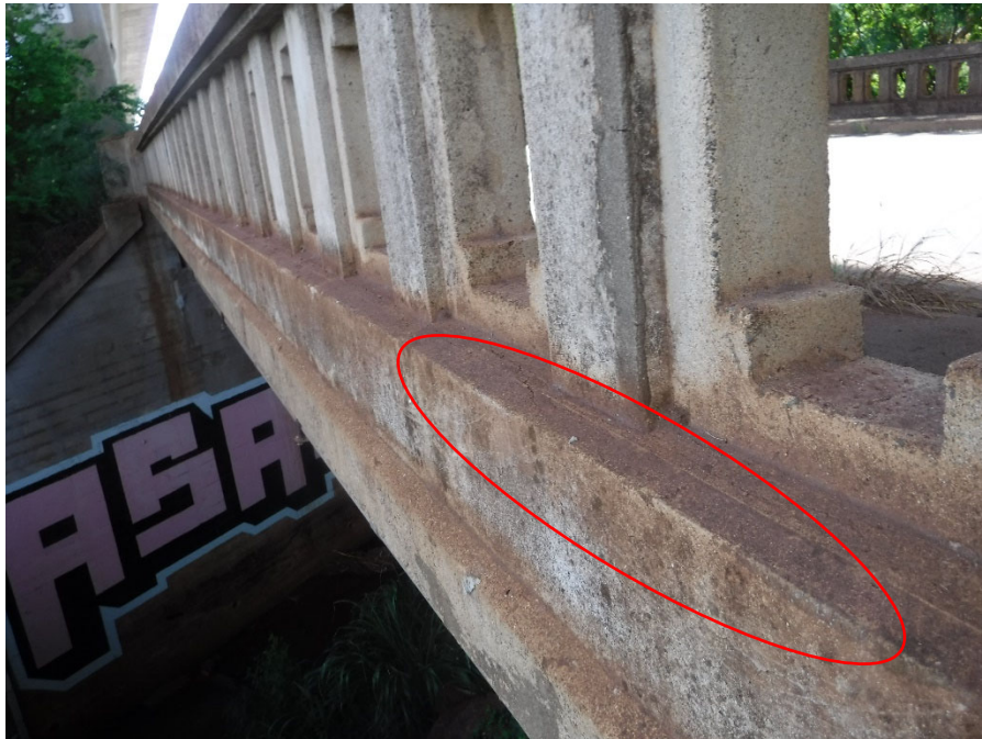
PHOTO 10 3'X4" DELAMINATION (3FT 1080 CS2) ON EXTERIOR FACE OF UPSTREAM BOTTOM RAIL NEAR WEST END OF BRIDGE
