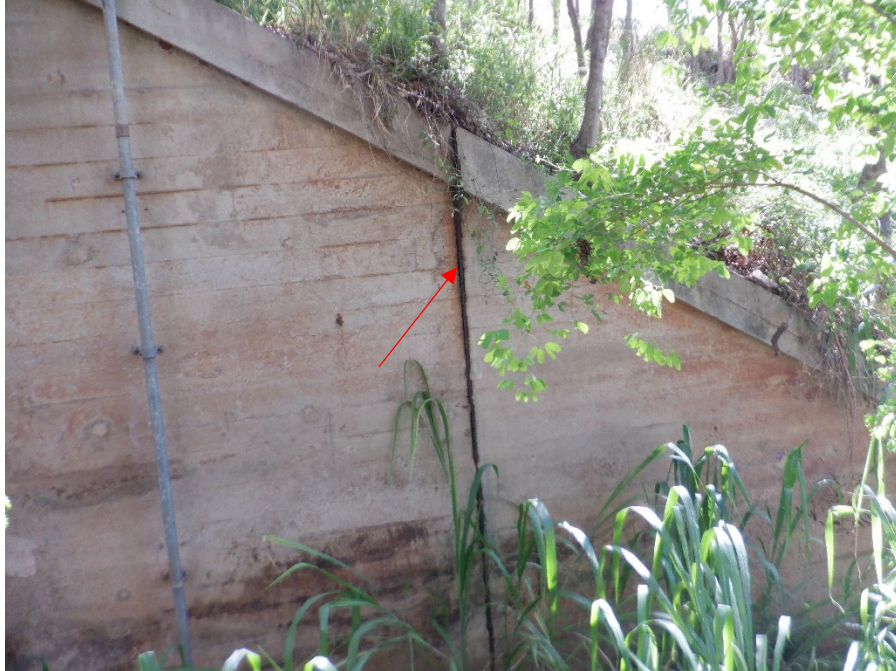
PHOTO 31 JOINT FILLER PROTRUDING FROM JOINT AT DOWNSTREAM EAST WINGWALL AND 1/2" GAP BETWEEN DOWNSTREAM EAST WINGWALL AND CHANNEL WALL
